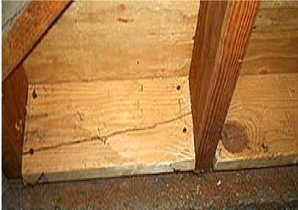
The photo above shows a block behind a shear wall that split with only four nails installed.
